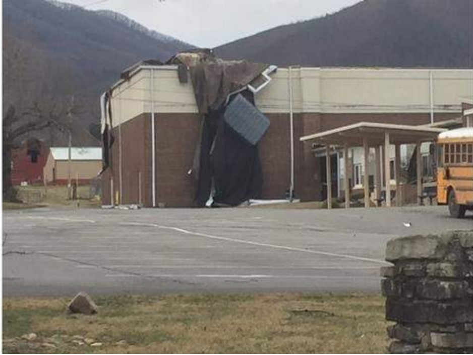
Roof damage to Camp Creek Elementary School in Greene County on January 23 rd [image via WHJL news]
